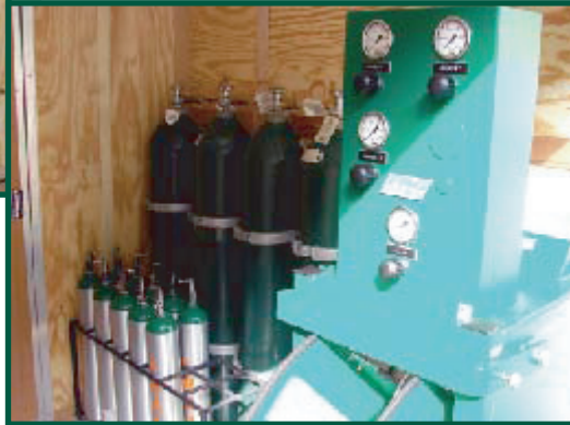
HYPRES fill containment, cascade and manifold.
